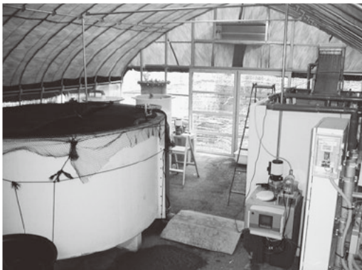
Fig. 1-2 Installation situation of the closed recirculating culture system.
